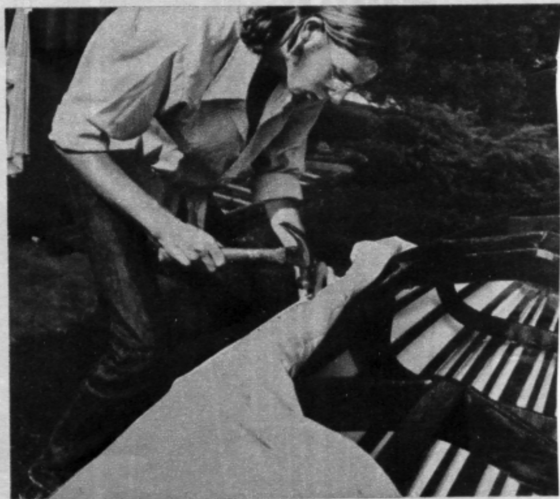
CANVAS hull sheathing is first attached along keel, then tacked to sheer clamps.
