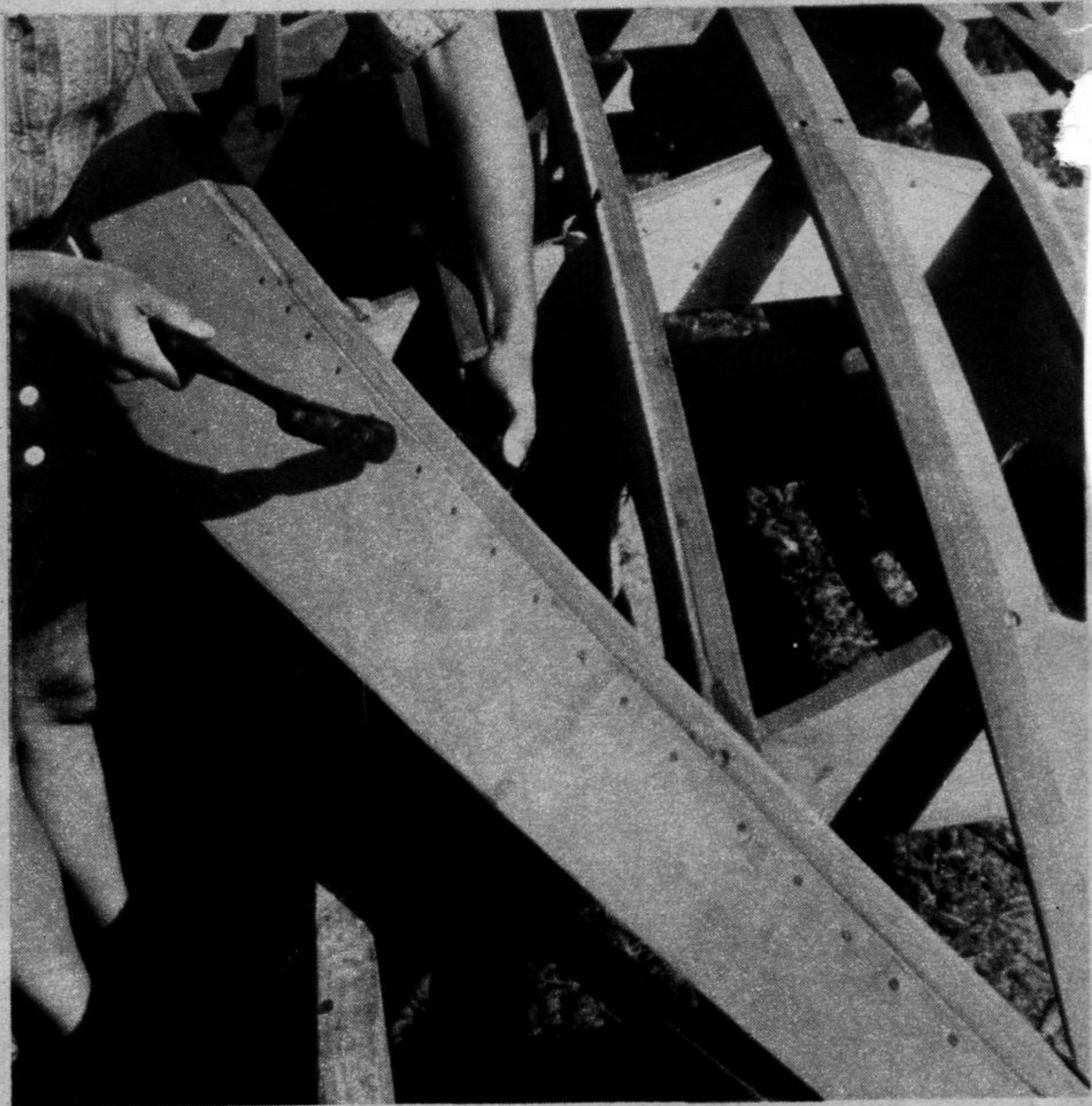
BOTTOM planking goes on with glue and nails. Use backing block for nailing. Note reinforcing blocks at rib/girder juncture.
