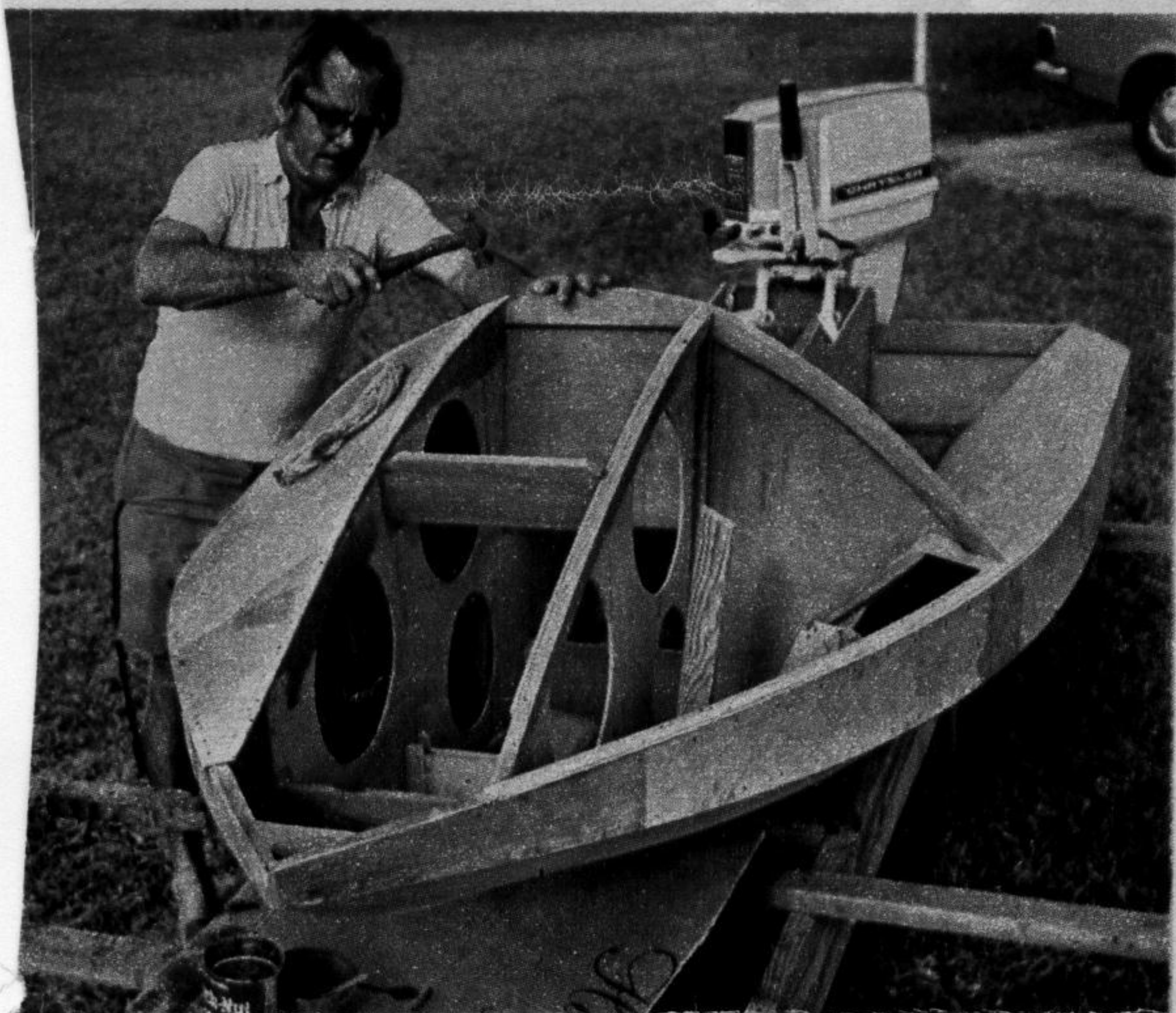
TAKE dashboard dimensions directly from the boat and fair in curve. Use template.
